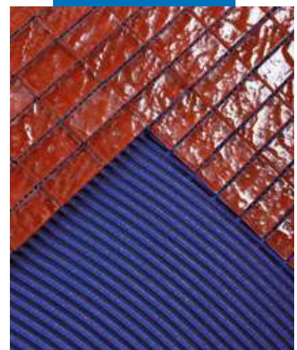
The following day, grouting with Kerapoxy Design in the same colour and the same application procedure previously shown
