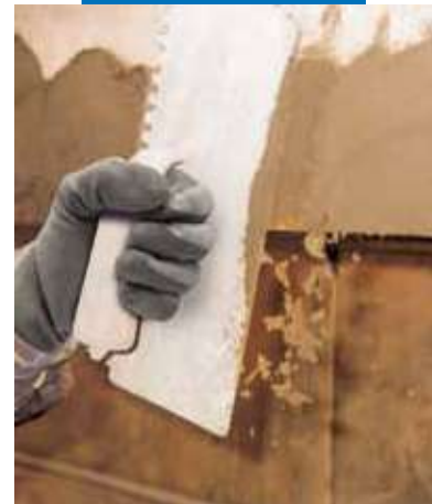
Restoring the front side of the concrete slab of a balcony: finishing
