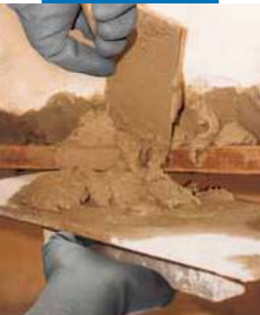
Restoring the front of the concrete slab of a balcony: applying Planitop 400
