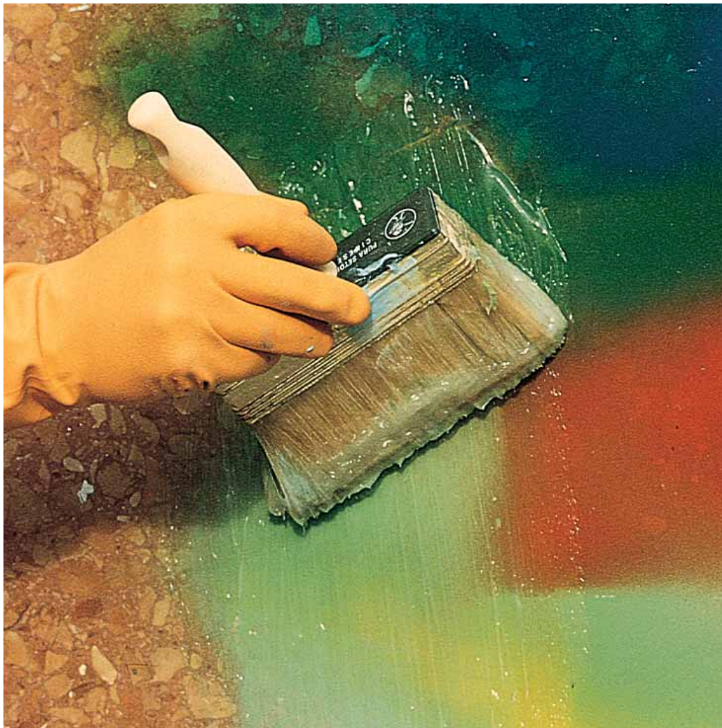
Rinsing graffiti away after scrubbing surface with WallGard Graffiti Remover Gel and brush
